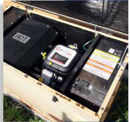
Guardian 15 KW Generator
