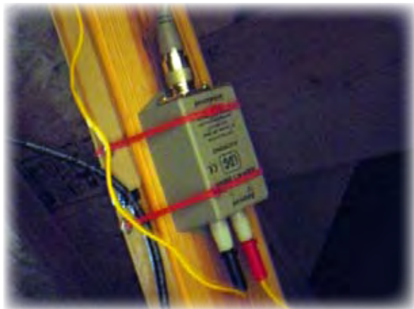
Detail of Balun Mounted to Roof Truss
