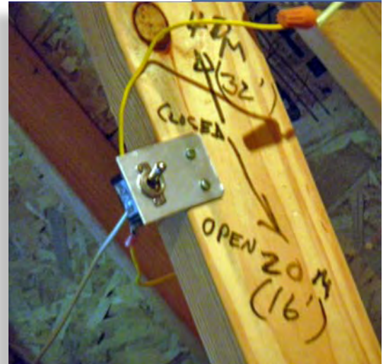
Attic Antenna Mounted to Roof Truss
