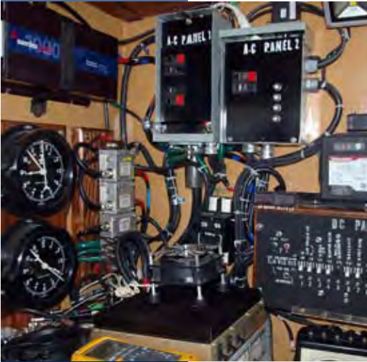
Genset Panel in Trailer
